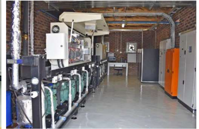
Image courtesy of https://energypartners.co.za/
