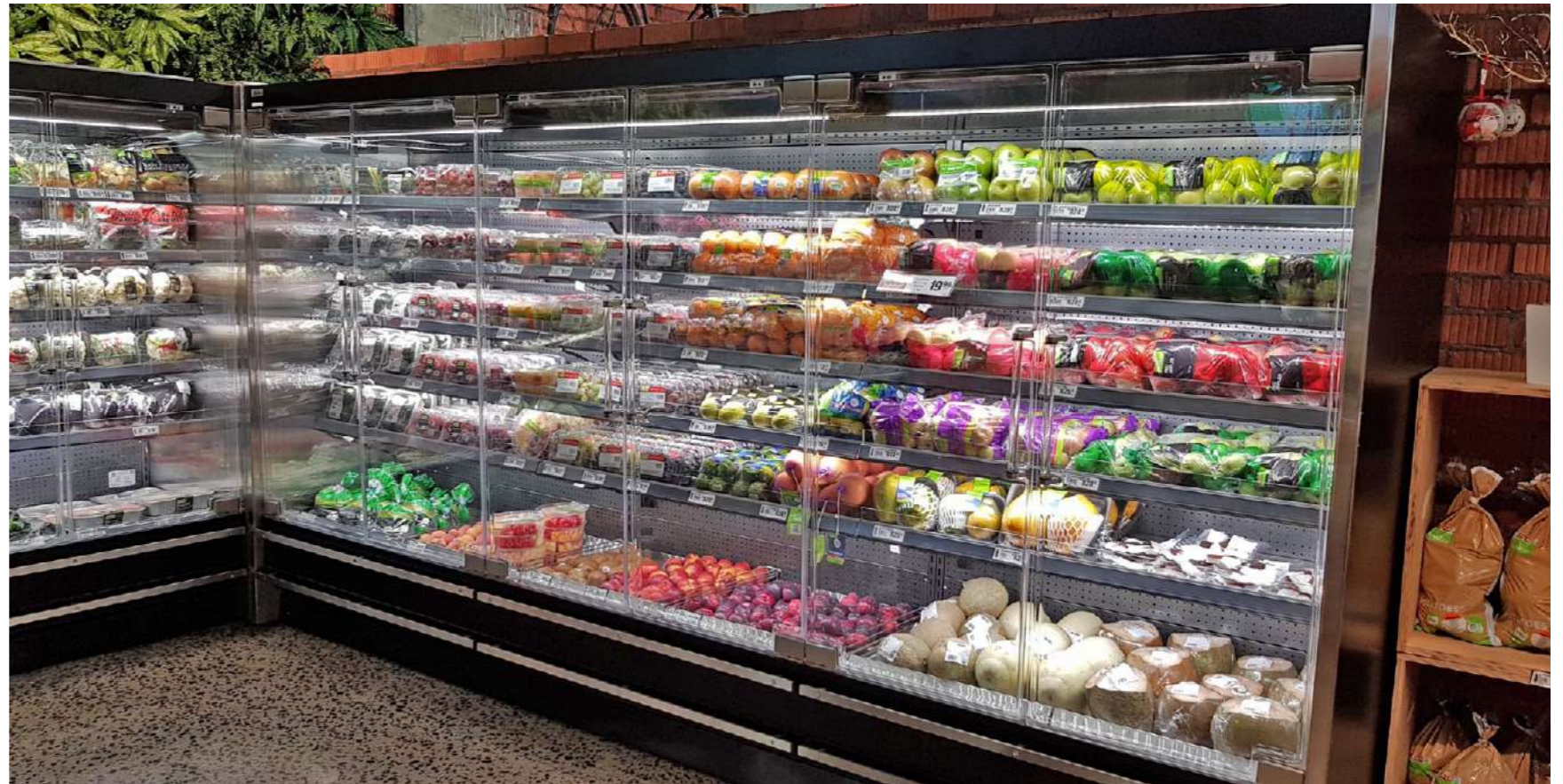
Energy efficient upright cabinet with acrylic doors, installed by Colcab in a Spar store in KwaZulu-Natal
